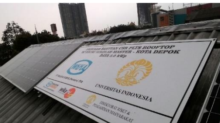
3 kWp Solar Rooftop
