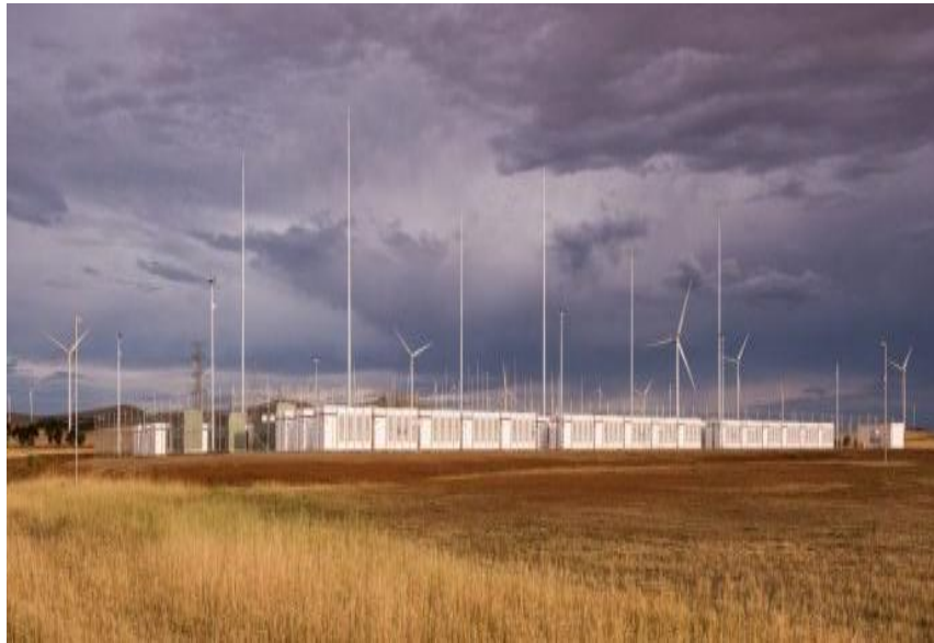
Tesla's facility at Hornsdale Wind Farm
